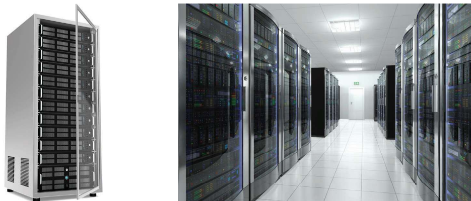
(a) A typical rack of servers (b) A typical server room in a data center
